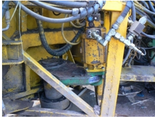
Figure 10- New hydraulic pump fitted.
