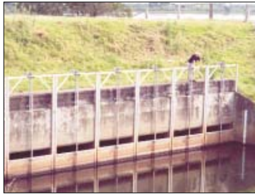
Figure 42. A large set of penstocks in a drain on the Clarence River floodplain. This set is located near the river levee on the floodgate headworks. Penstocks can be used to retain water in the drain. (Photo: Rob Lloyd)
