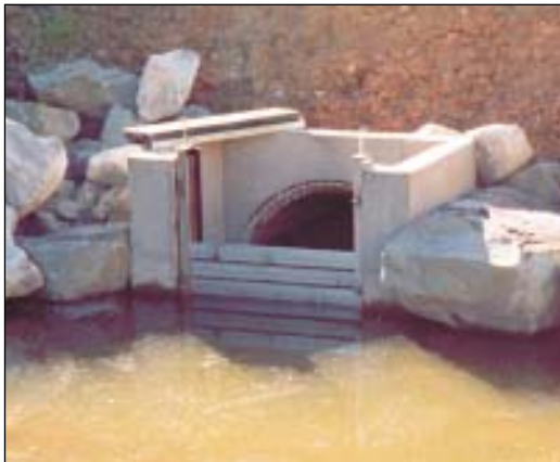
Figure 43. dropboard culverts are a simple way to retain water to a desired level. Leaving a space between the boards and the pipes helps provide better drainage of overtopping waters. (Photo: Rob Lloyd)
