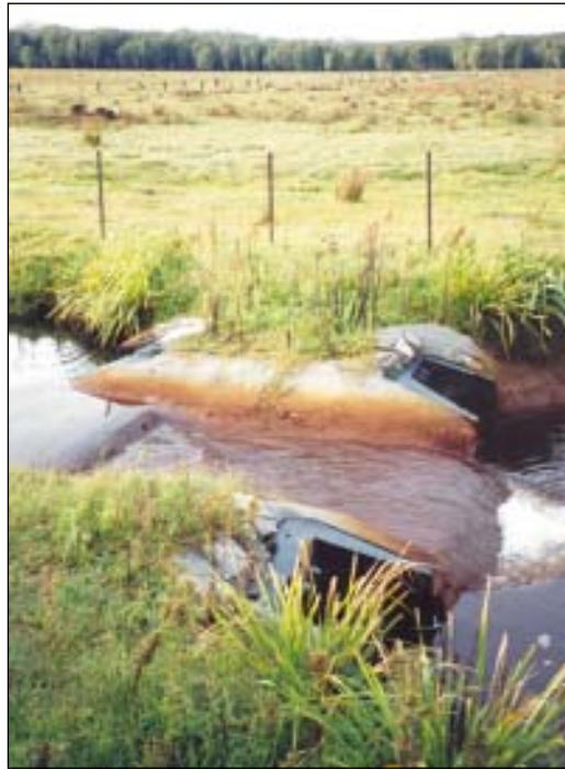
Figure 44. Weirs provide more permanent water retention. This one is used to maintain high drain water levels and reduce acid groundwater seepage.
