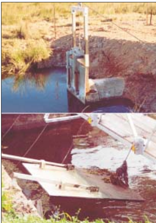
Figure 23. Vertical winch gates (above) and horizontal winch gates (below). Both are opened via a cable and pulley system attached to a stationary winch on the bank. (Photos: Rob Lloyd and Alan Cibilic)
