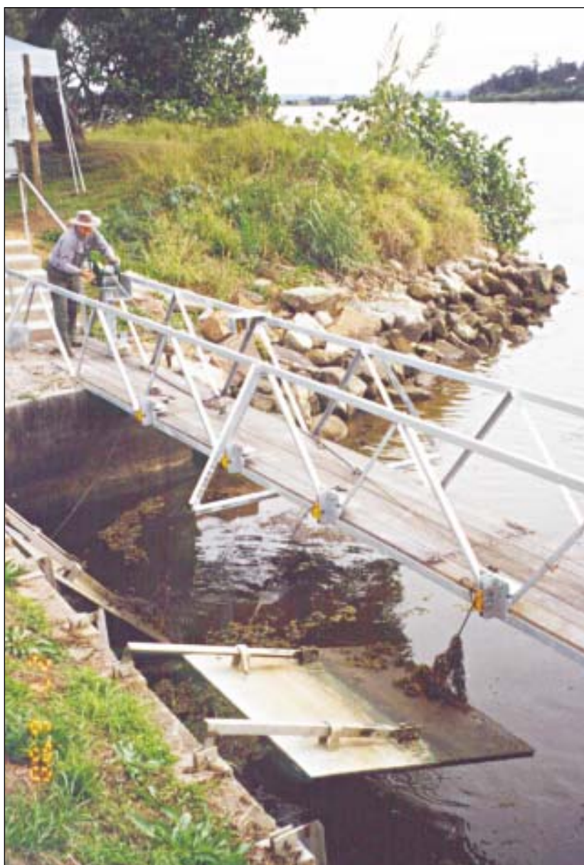
Figure 53: Opening up floodgates using a horizontal winch system on a drain in the Clarence River. Floodgate opening devices and opening strategies should be tailored to suit management objectives and the characteristics of individual drainage systems. (Photo: Alan Cibilic)
