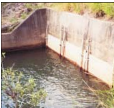
Figure 5. Floodgates set in a concrete culvert headwall - a common sight on coastal floodplains. Floodgates allow drainage outflow, but prevent inflow of salt water or floodwaters. (Photo: NSW Agriculture)
