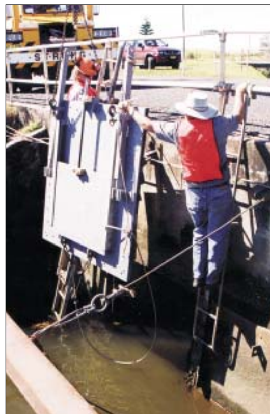
Figure 56. Installing sluice gates on the Empire Vale drainage system. Selecting drain system management methods should be based on clear objectives and a sound understanding of the key features of the drainage system (see pg 14). The concerns of all stakeholders need to be considered. (Photo: Jon Woodworth)
