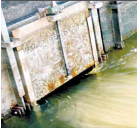
Figure 22. River water flowing through an open sluice gate. This one operates with a worm drive mechanism. (Photo: Michael Wood)
