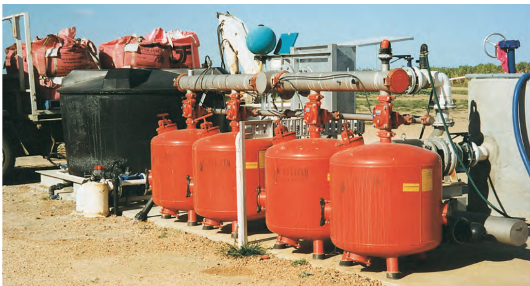
Figure 12. Large sand filters for drip irrigation.
