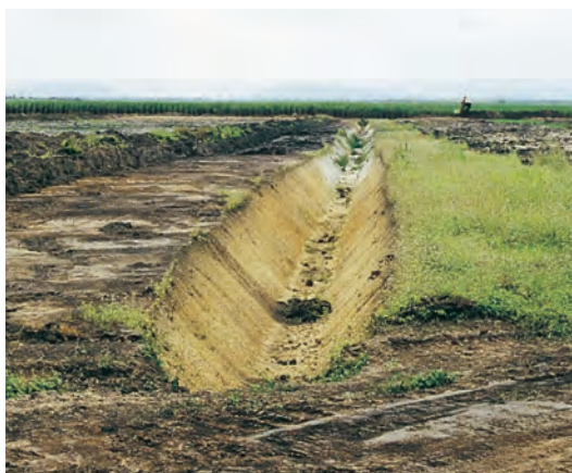
Figure 8. Deep open drains are only suitable for flat lands and stable soils that do not have an acid sulfate potential.
