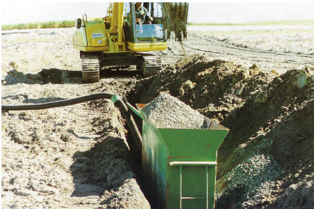
Figure 9. Gravel hopper in an excavated trench for placing a gravel envelope around corrugated drainage pipe.
